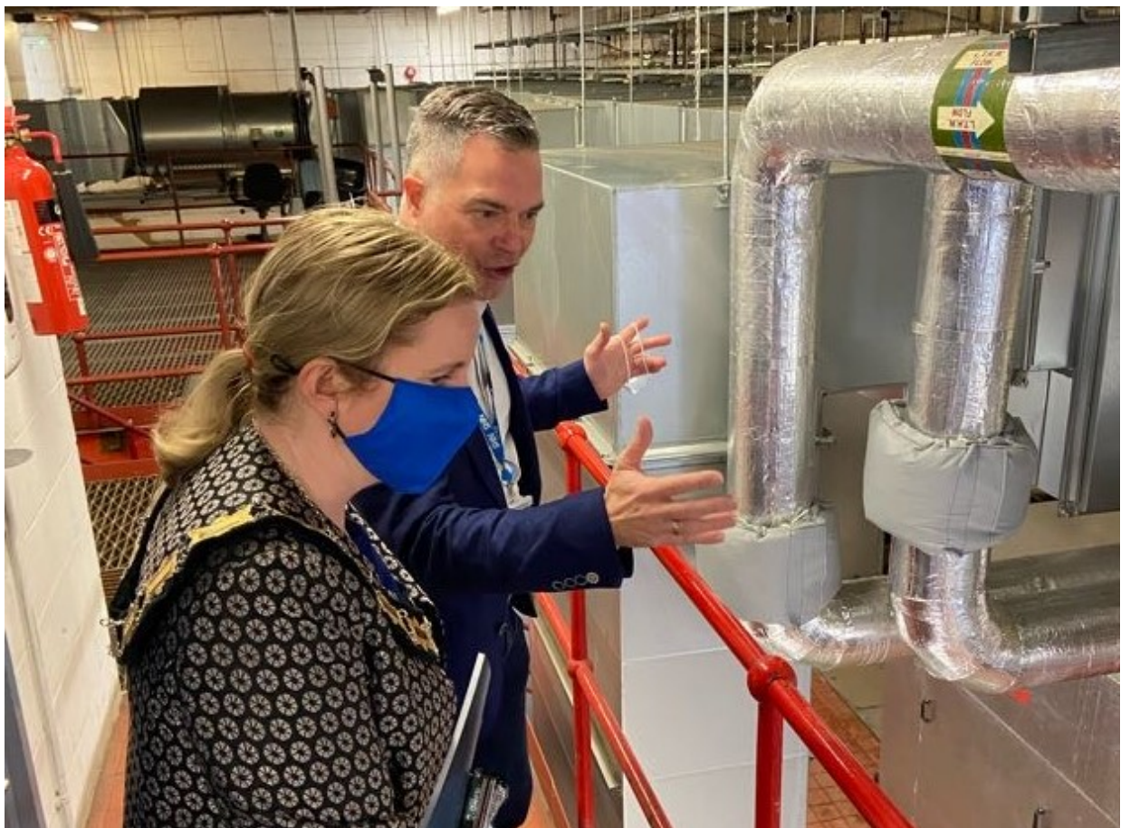
Guy Kieser, Associate Director of Estates at RBH, pictured here with the Mayor of Reading, Cllr Rachel Eden, being shown the complex boiler systems which heat the hospital
